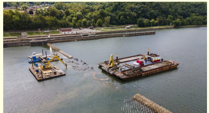
Contractors for the Pittsburgh Engineer District use floating barges to drill, demolish and remove rubble from the former Monongahela River Dam 3 in Elizabeth, Pa., on August 2, 2024, creating a 100-foot channel. (Photo by Michel Sauret/ Pittsburgh Engineer District)
